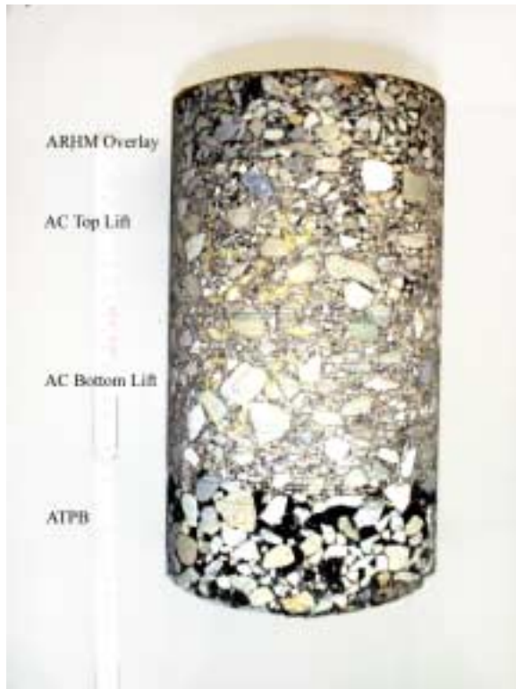
Figure 8. Core from Section 543, station 13 outside the trafficked area showing ATPB still intact.
