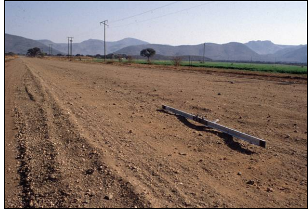
Figure 7: Washboarding and raveling.
