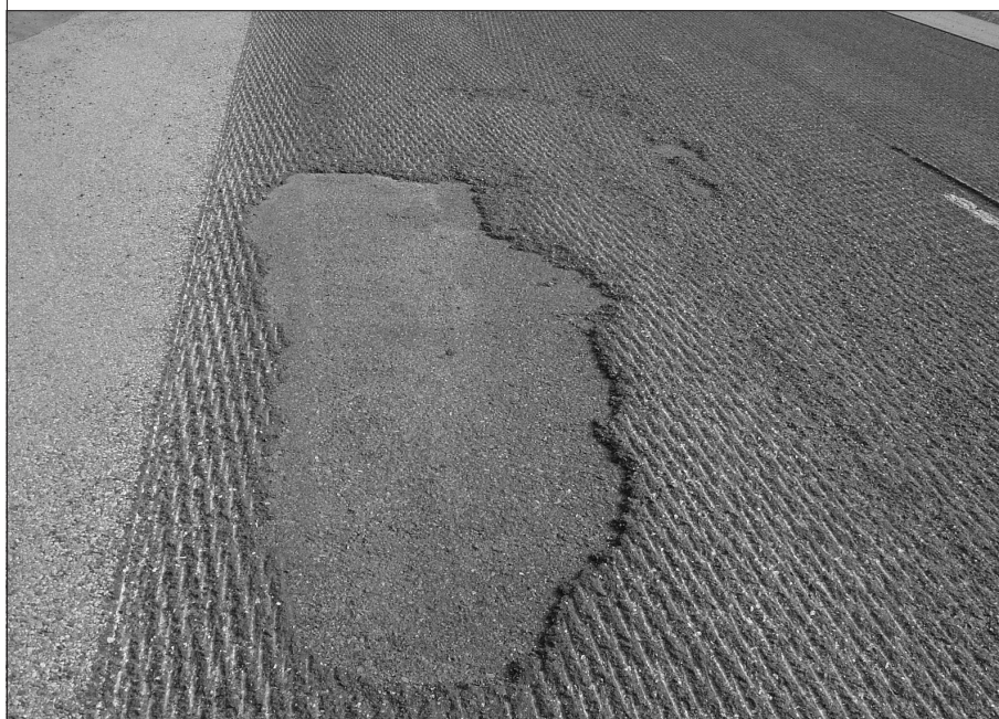
FIGURE 1 Debonding between pavement layers
