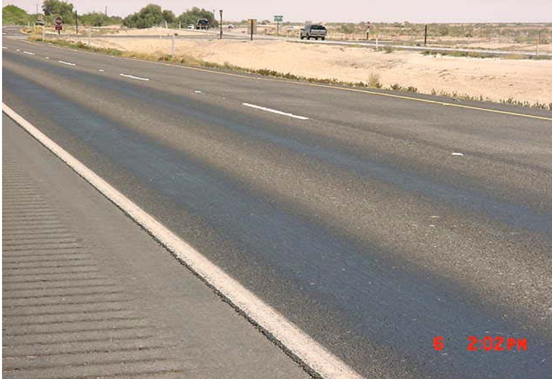
Figure 6. First post-construction inspection showing rutting in northbound #2 lane, March 2004 (Caltrans Maintenance – Ron Jones).
