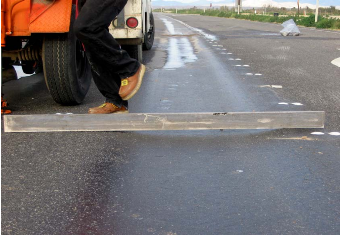
Figure 8. PRC site visit showing 33-mm rut and bleeding, January 2005 (Station 616+21, northbound #2 lane).
