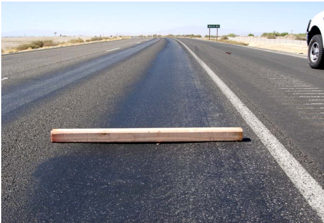
Figure 7. Second post-construction inspection showing rutting in northbound #2 lane, September 2004 (Caltrans Maintenance – Ron Jones).
